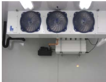
Controlled Environment Evaporator, shown here with Ultrasonic Humidifier
